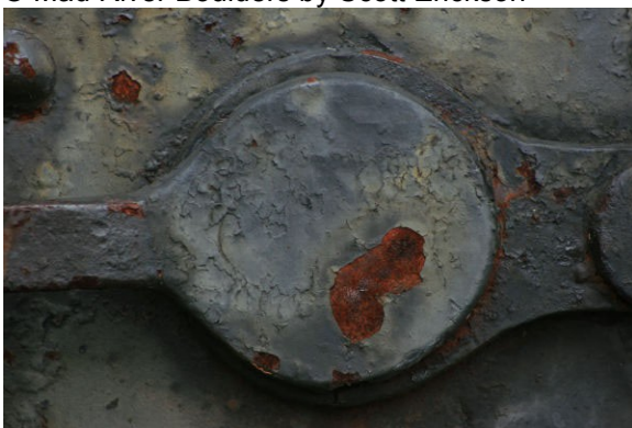
© Corrosion by Barbara Lippert
